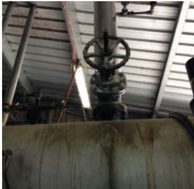
FIGURE 11: CONTROL VALVE ON TOP OF BOILER
