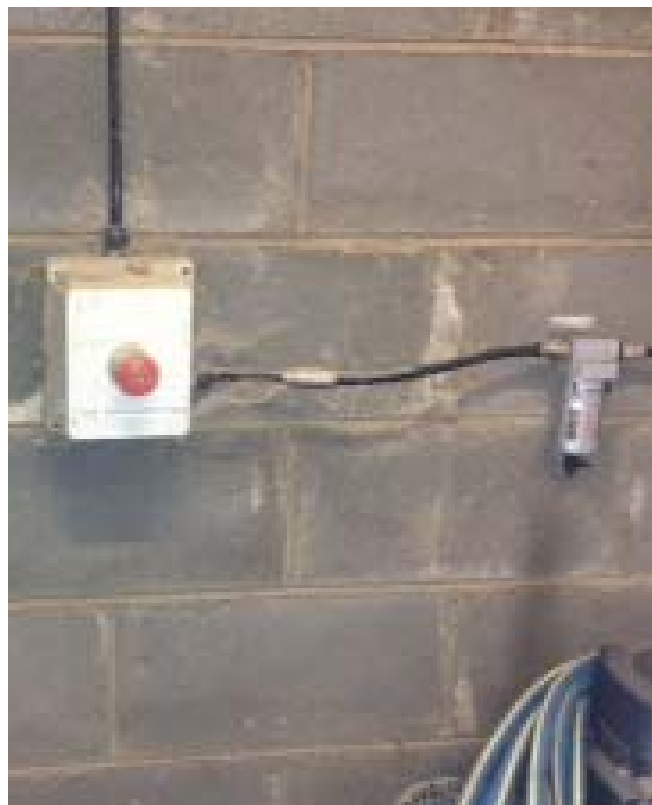
FIGURE 9: CONTROL PANEL IN FEEDMILL BOILER ROOM (EMERGENCY STOP)
