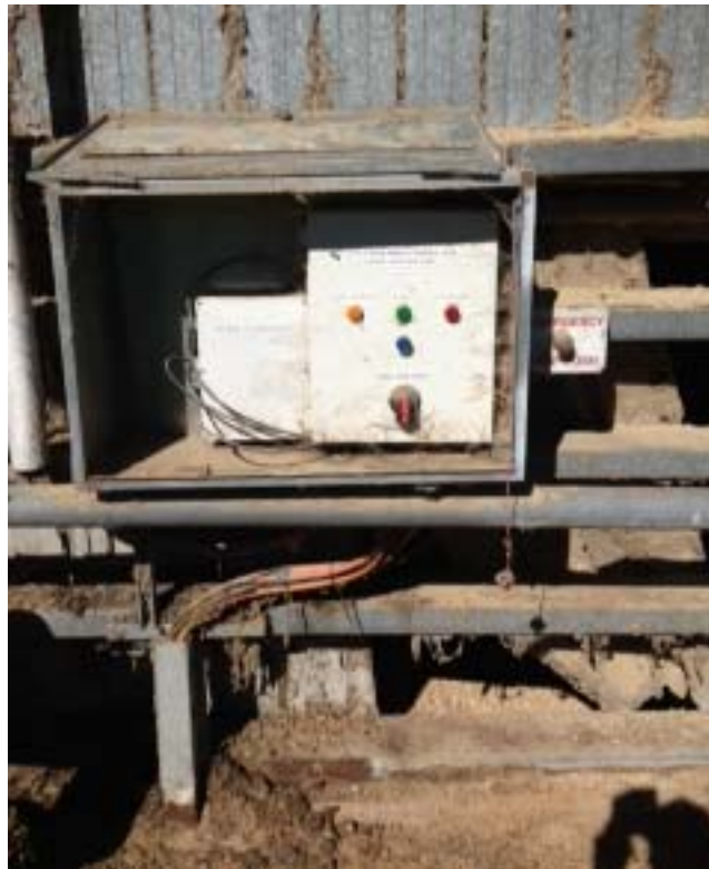
FIGURE 8: CONTROL PANEL IN COMMODITY SHED
