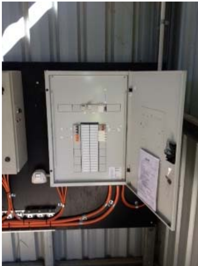
FIGURE 4: ISOLATION SWITCH IN THE PUMP SHED AT TURKEYS NEST
