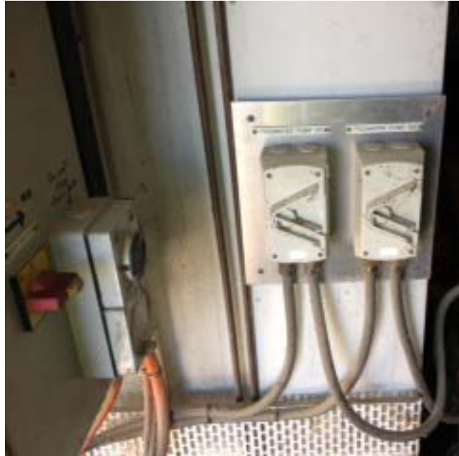
FIGURE 10: CONTROL SWITCHES ON SIDE OF BOILER
