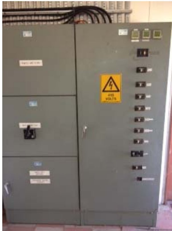
FIGURE 5: POWER SWITCH IN HOPPER CONTROL ROOM
