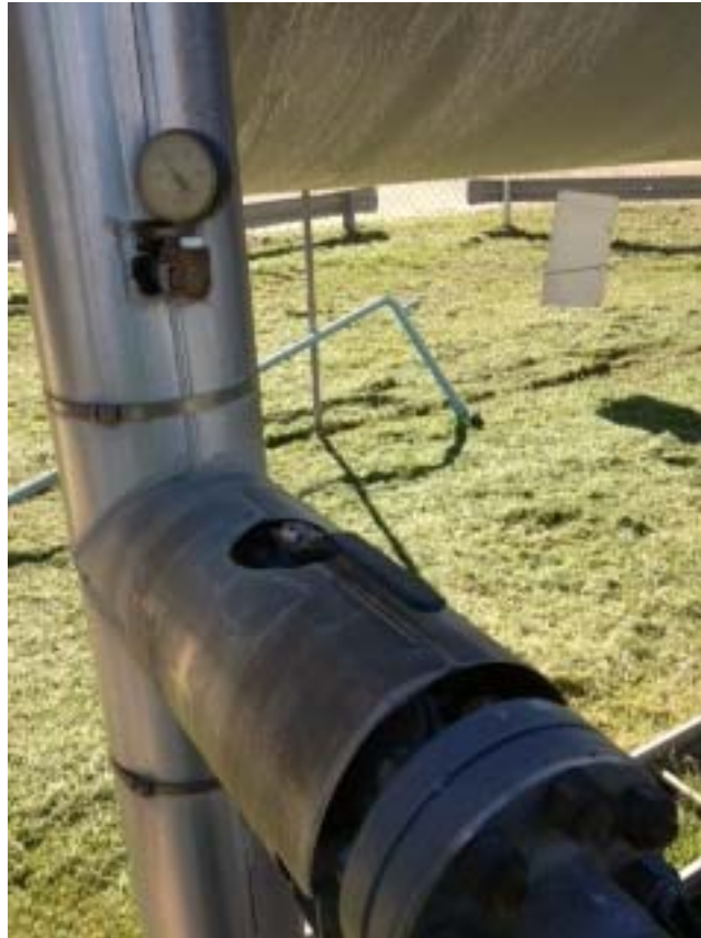
FIGURE 7: LPG TANK CONTROL VALVE
